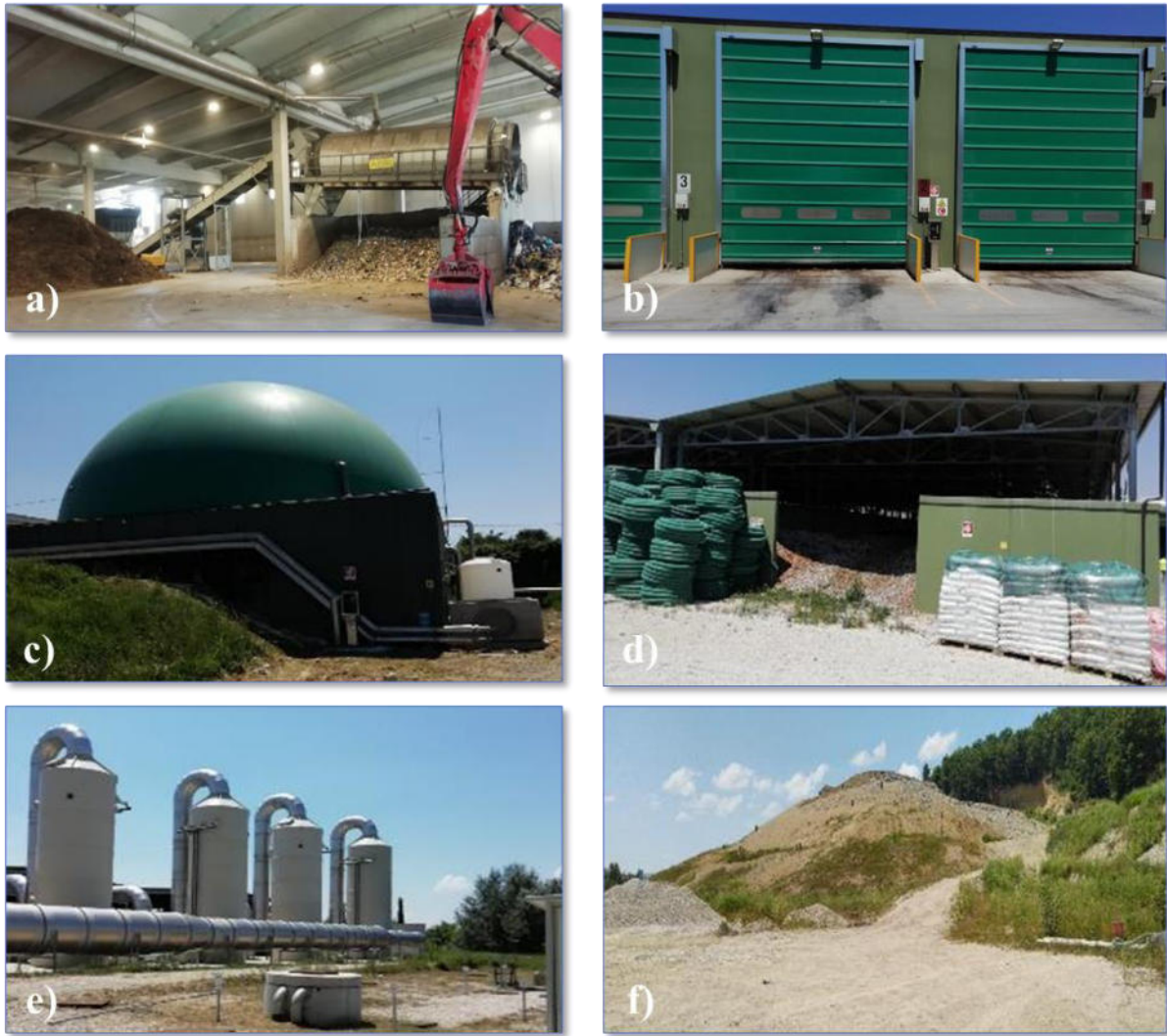
Fig. 2-2. Pictures of the different sections in the facility. a) MBT unit, b) anaerobic digesters, c) volumetric dome, d) aerobic stabilisation shed, e) scrubbers and f) sanitary landfill.
